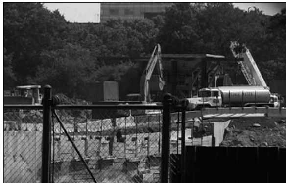
Man's Way of Producing Safe, Clean Water (Construction of Water Treatment Plant in Van Cortlandt Park)
